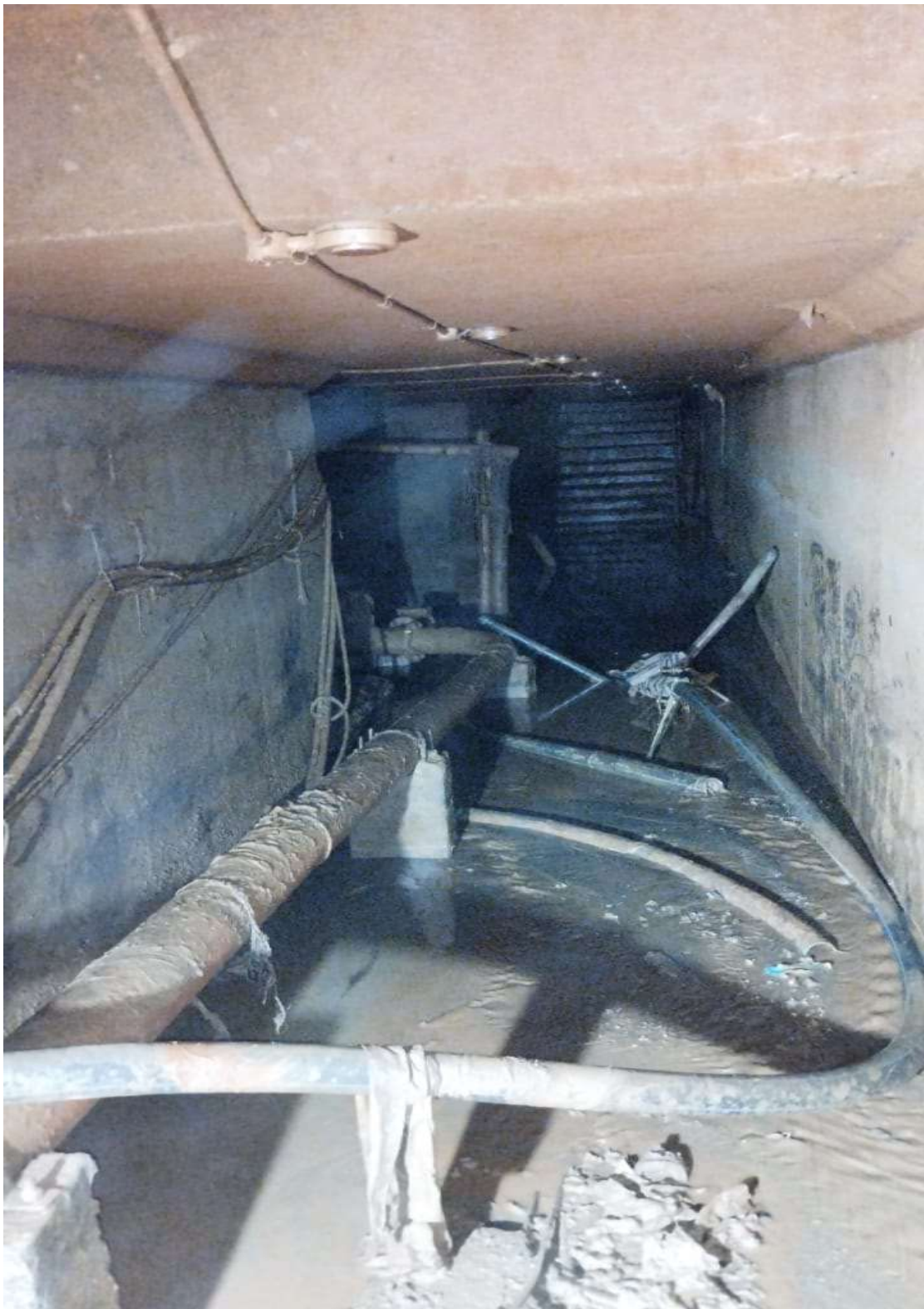
Existing dewatering pipeline inside Dam gallery
